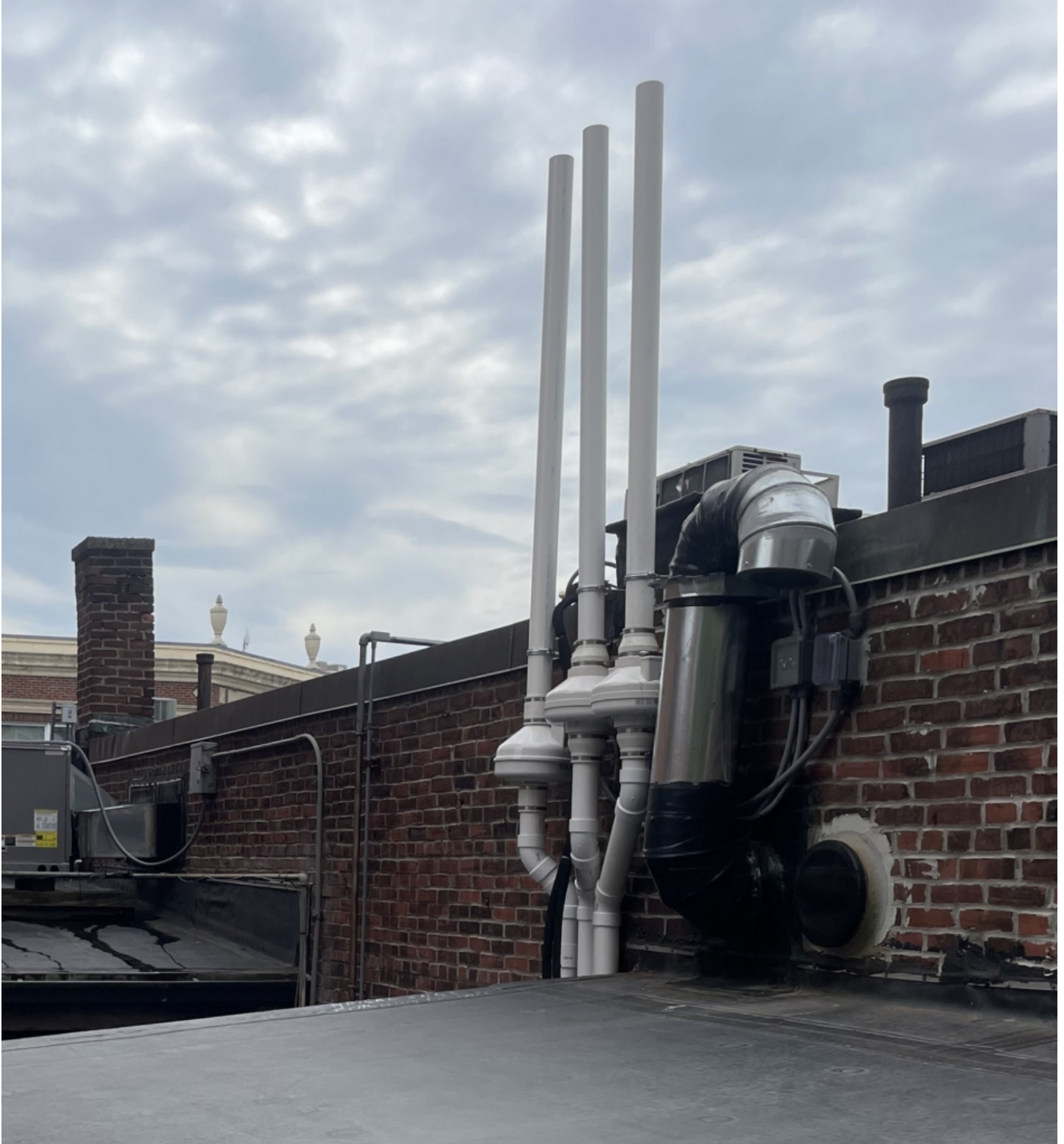
Photo of an active vapor intrusion system in-situ
